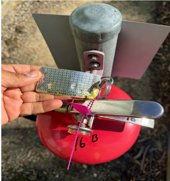
Fire extinguisher tested
