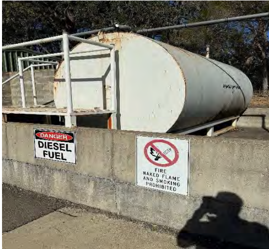
Diesel fuel tank bunded
