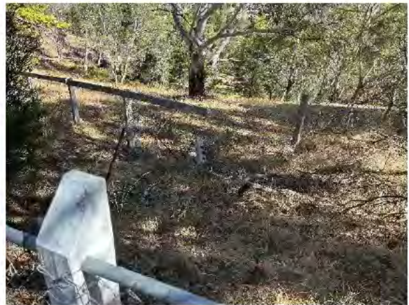
Photo 2: Fence Damage, Montacute Cemetery
